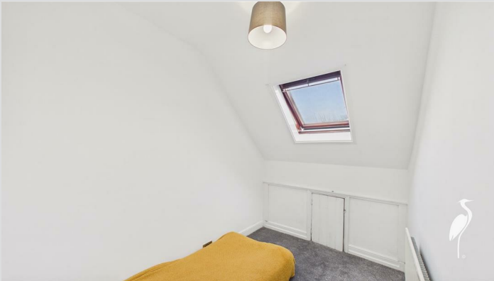
Velux window and radiator.
