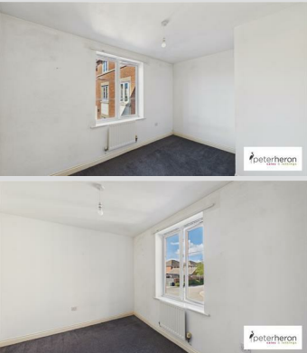
Double glazed window and radiator.
