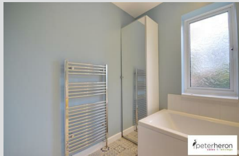
Contemporary suite comprising of a low level WC with concealed cistern, pedestal basin and P shaped bath with
